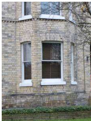
Cracking above and below bay window to No. 78 Ashley Road
